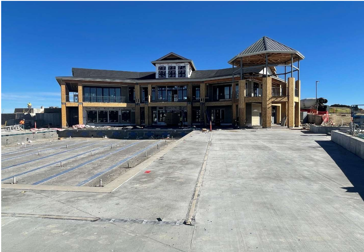
Rec Center – Windows installed, roofing complete, and Concrete Pool Deck almost complete
