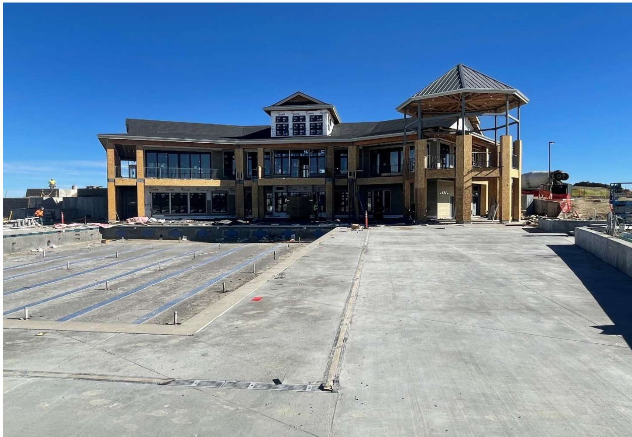
Rec Center – Windows installed, roofing complete, and Concrete Pool Deck almost complete
